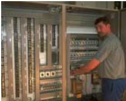
Functional test of secondary installation
